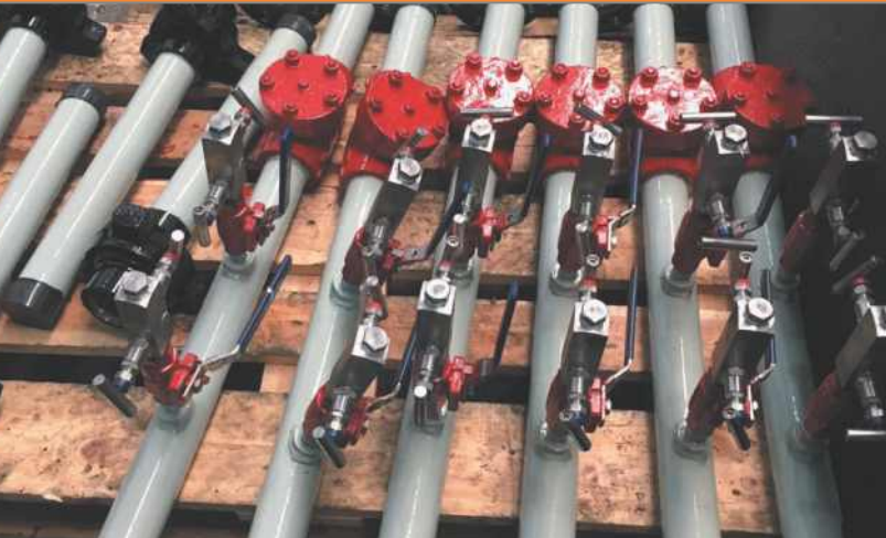
puentes de shale shale manifolds / manifolds de shale
